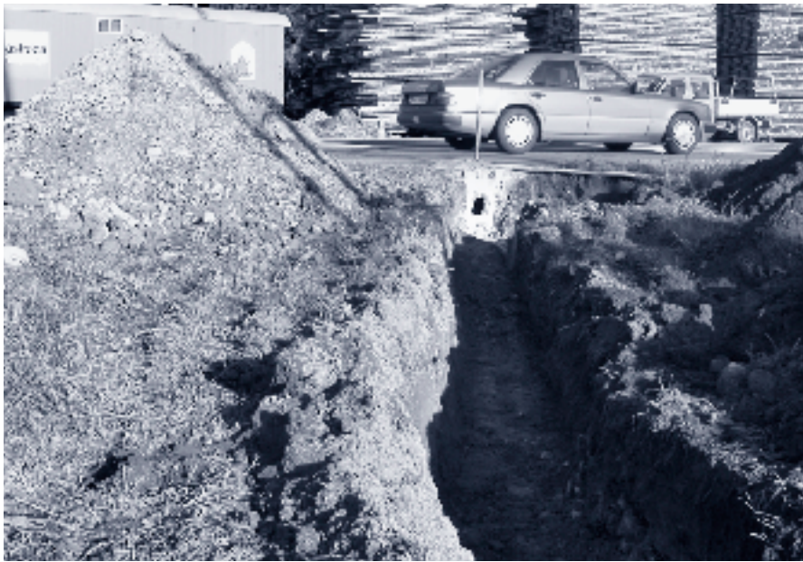
Fig. 3: Connection of the road runoff with the test facility.
