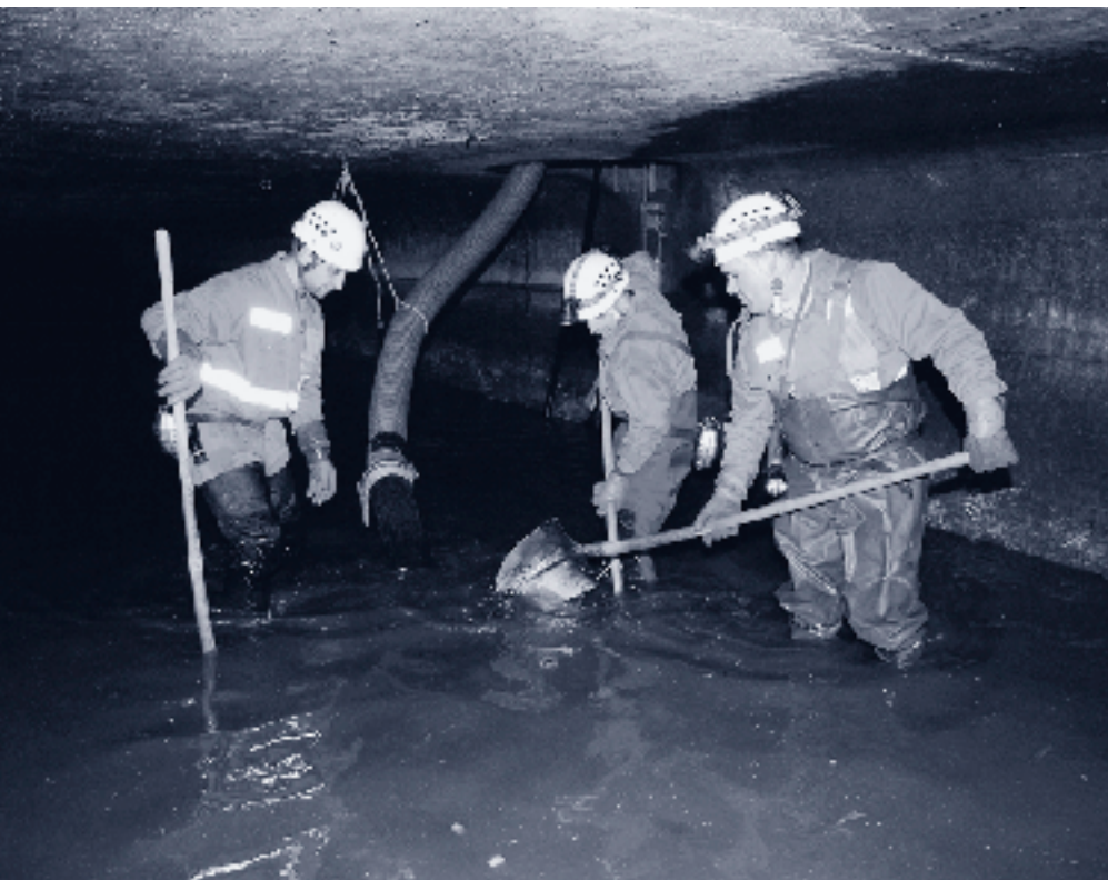
Maintenance work in the sewer system by employees of "Entsorgung + Recycling Zurich".
